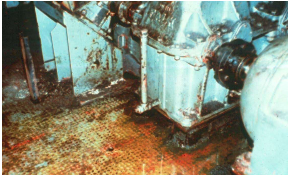
Figure 16.2.61 Cracked Speed Reducer Housing
