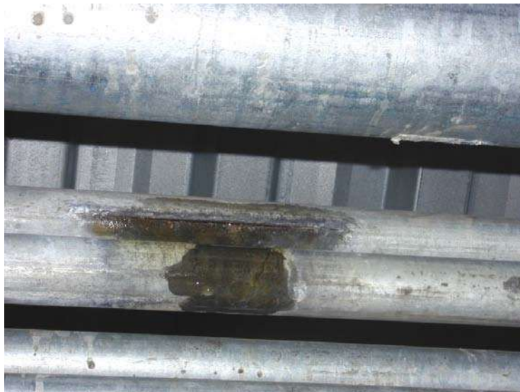
Photo No.14 Conduit , Span 3 – note conduit is split and leaking water
