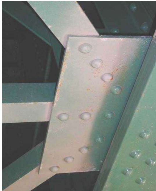
Photo No.18 Lateral bracing connection between beam #3 and #4, in span 2 – note no final paint coat, and rust freckles
