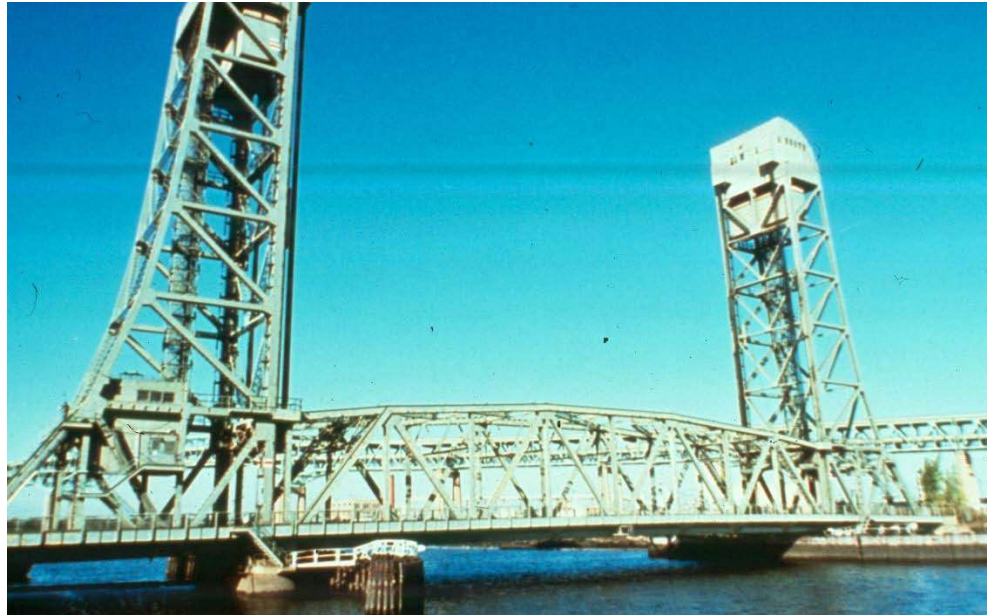
Figure 16.2.18 Vertical Lift Bridge with Power and Drive System on Towers
