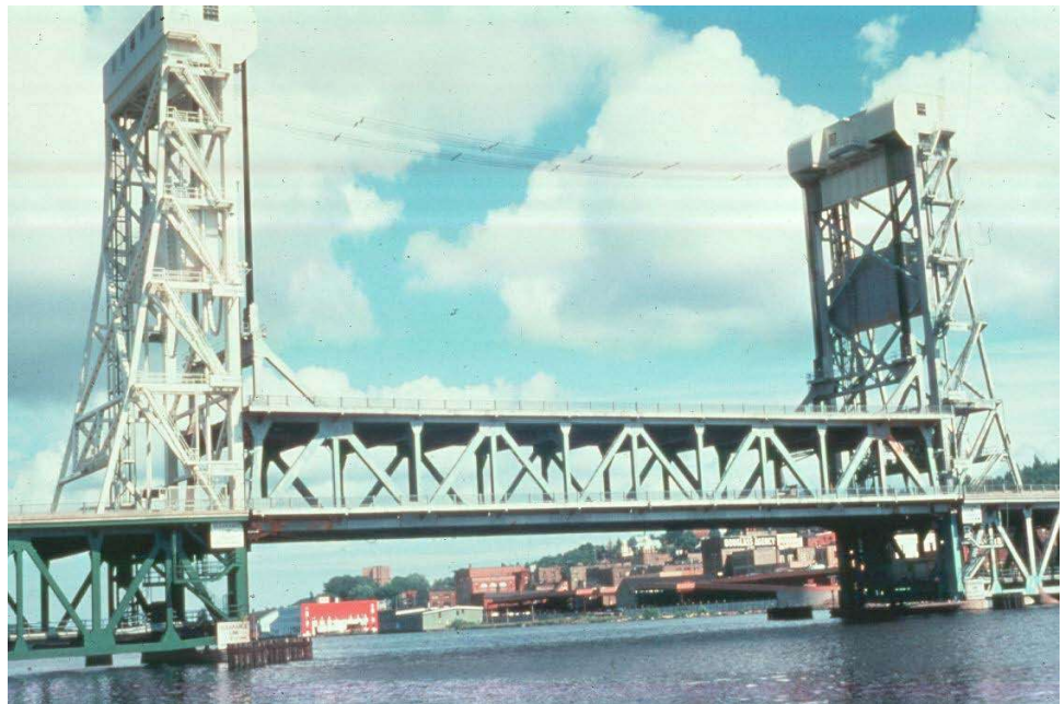
Figure 16.2.33 Concrete Counterweight on a Vertical Lift Bridge
