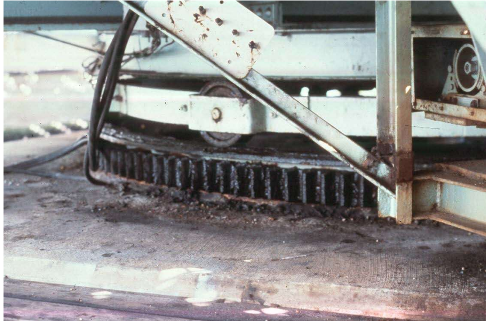
Figure 16.2.37 Balance Wheel in-place over Circular Rack
