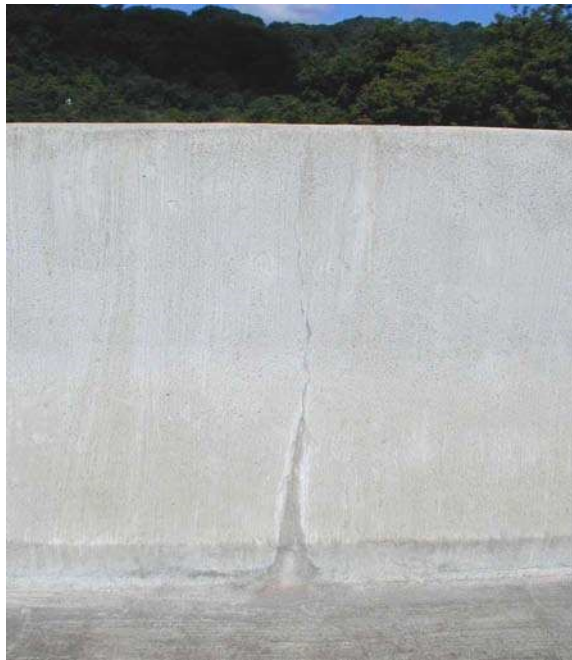
Photo No.16 Typical parapet crack
