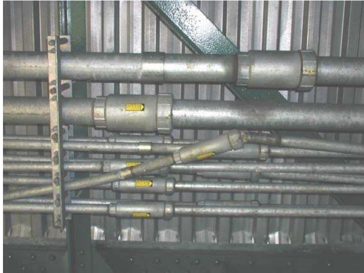
Photo No. 13 Conduit and Couplers, Span 1 – note bend in conduit, and coupler separation
