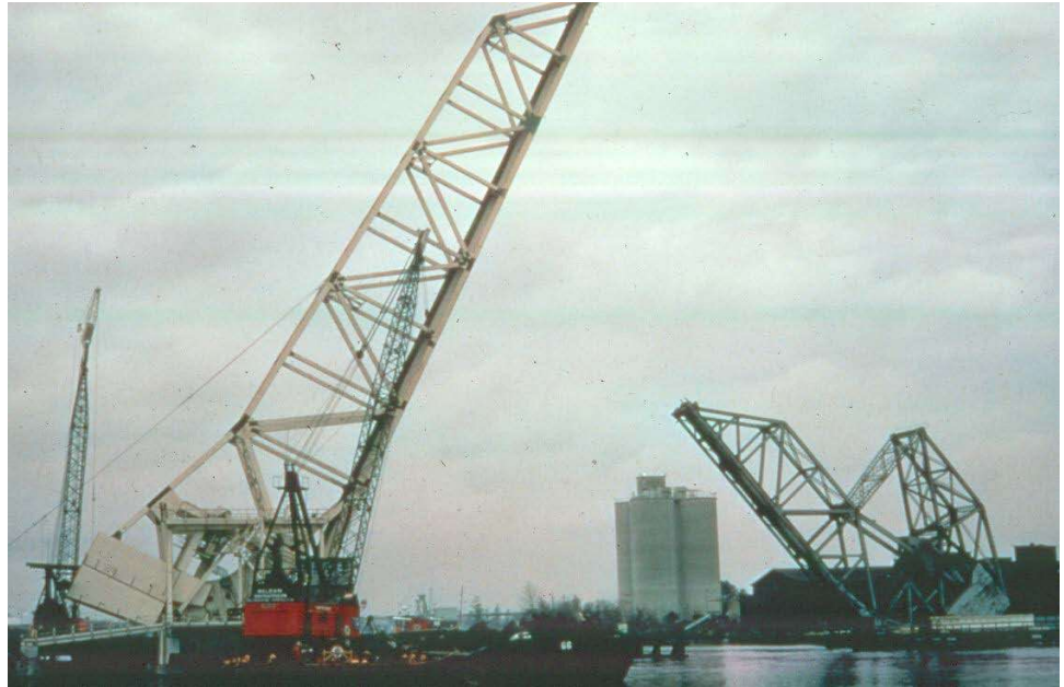
Figure 16.2.32 Concrete Counterweight on a Single-Leaf Bascule Bridge
