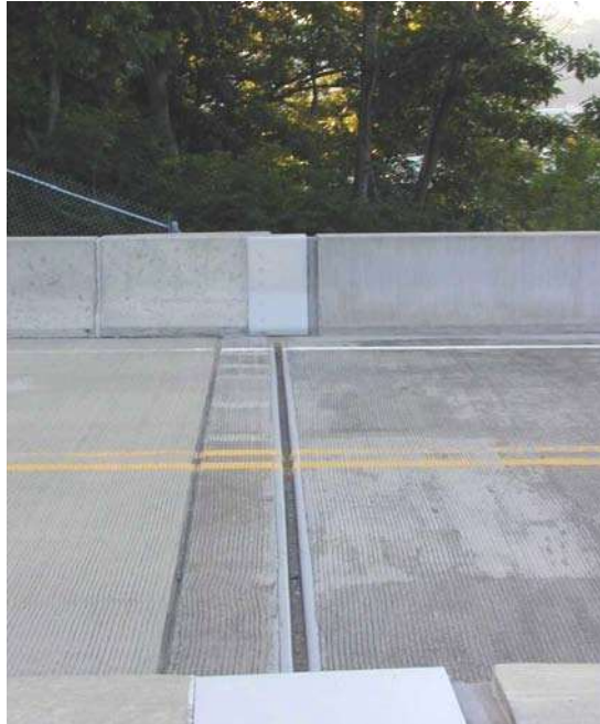
Photo No. 17 Strip Seal at North Abutment (typ.) – note minor debris accumulation
