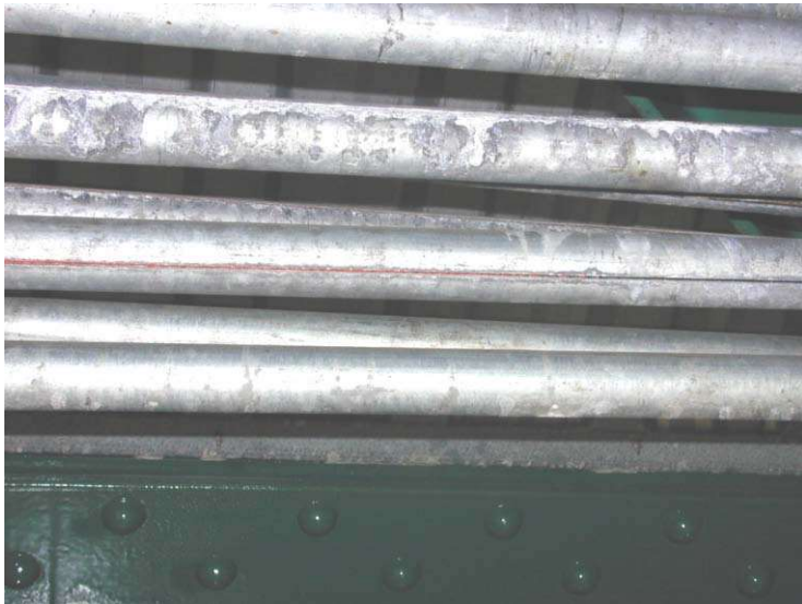
Photo No. 12 Conduit, Span 1 – note longitudinal crack/split
